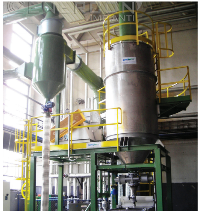
■ Suction and wet filtration plant from shot blasting operations - Slovakia
