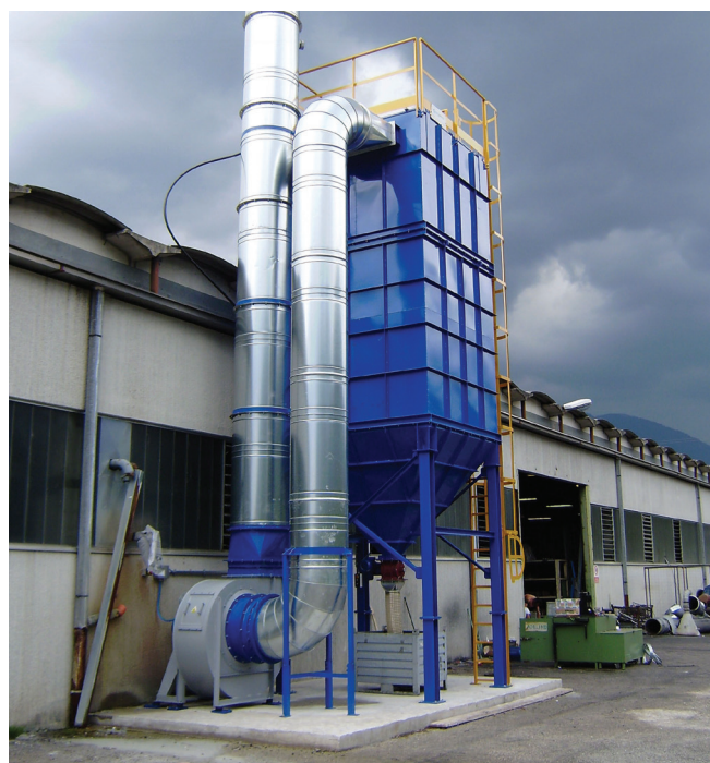
■ Fume suction and filtration system (flow rate 20,000 m 3 /h) for aluminum smelting furnaces - Italy
