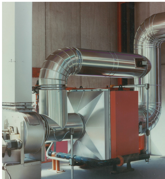
■ Fume/water heat exchanger for the use of heated water inside the plant - Italy
