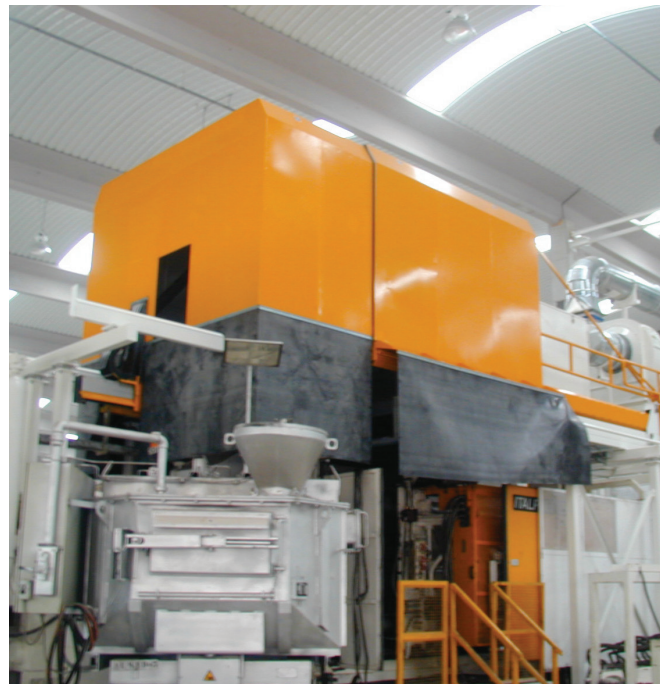
■ Hood into two parts complete with ENERPRESS filtration system, fan and individual expulsion into the atmosphere on ITALPRESSE IP1650 die-casting machine - Spain
