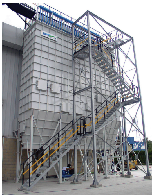
■ Suction and filtration system for dusts - Spain
