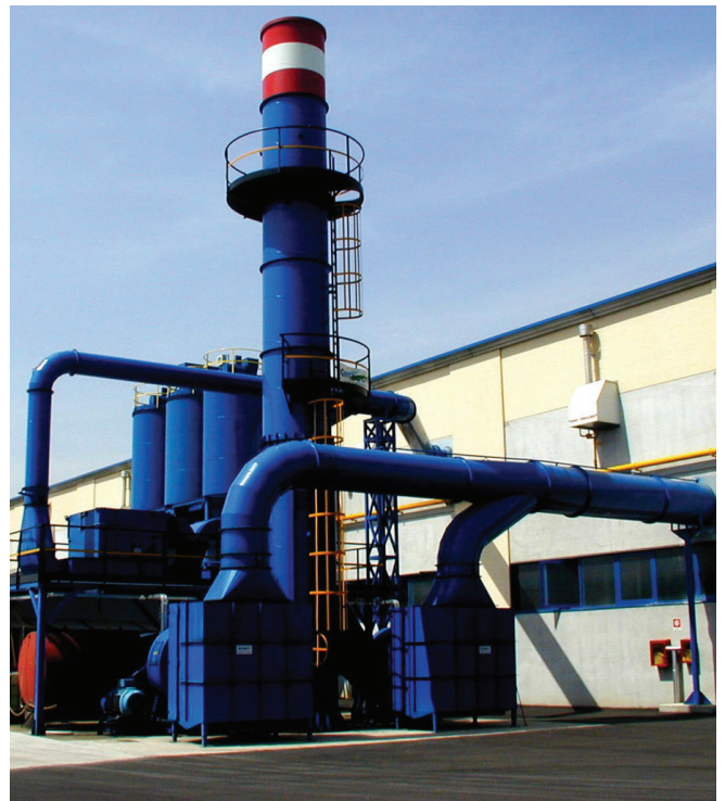
Centralized suction and filtration system ENERPROG - Italy
