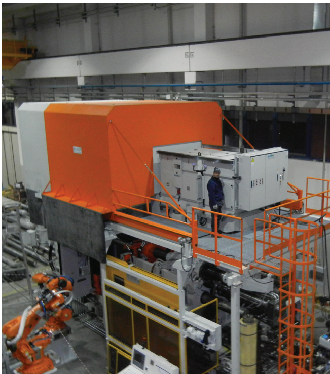
■ Hood into two parts complete with individual ENERPRESS suction and filtration system for recirculation of purified air in a die-casting machine - Russia
