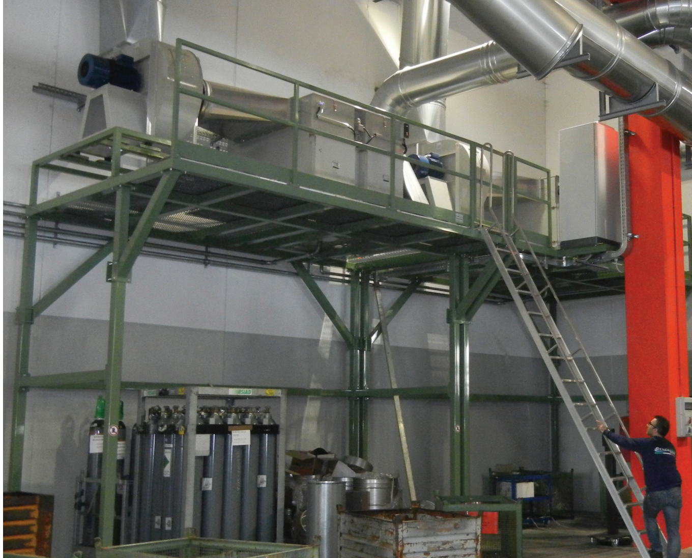
ENERPRESS filters on independent supporting structures dedicated to die casting machines with fans and expulsion chimneys. Italy
