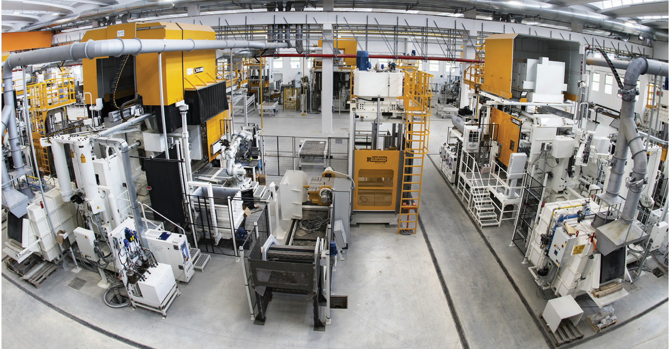
Two parts hoods on die casting machines complete with ENERORESS filters, extraction fans and expulsion chimneys - Italy
