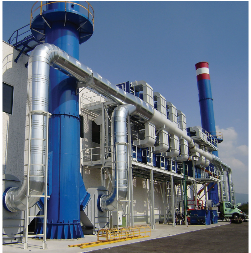
ENERPROG centralized suction and filtration system in 12 modules for a total suction flow of 200,000 m 3 /h dedicated to 22 presses - Italy
