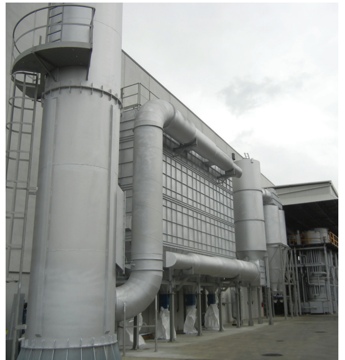
■ Fume suction and filtration system from aluminum melting furnaces with chemical treatment of the fumes in the reactor and reagent storage and dosing system - Italy
