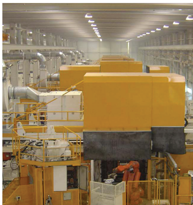
■ Die-casting machines with hoods in two parts complete with ENERPRESS filters, fans and individual chimneys for the expulsion of air purified in the atmosphere - Spain
