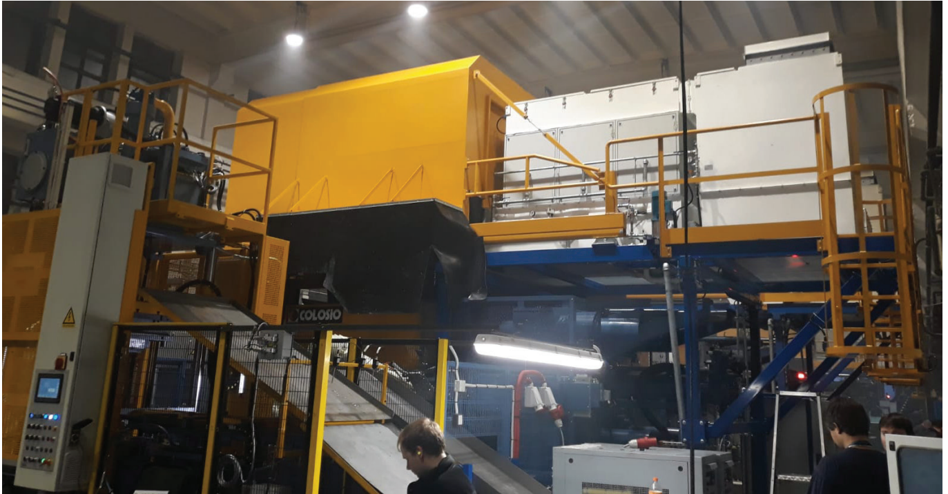
■ Hood into two parts complete with ENERPRESS suction and filtration system for recirculation of purified air in a COLOSIO PFO1000 die-casting machine - Czech Republic
