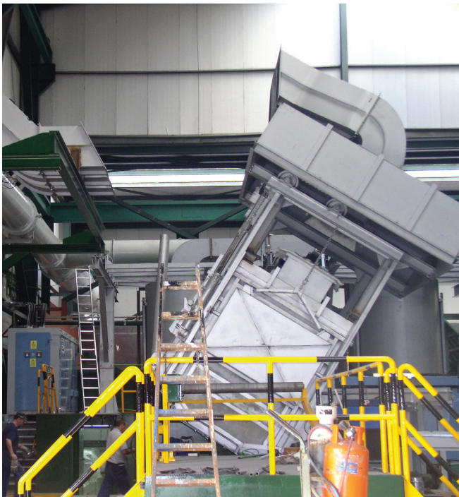
■ Extraction hoods on combustion opening of rotating aluminum smelting furnaces - Spain
